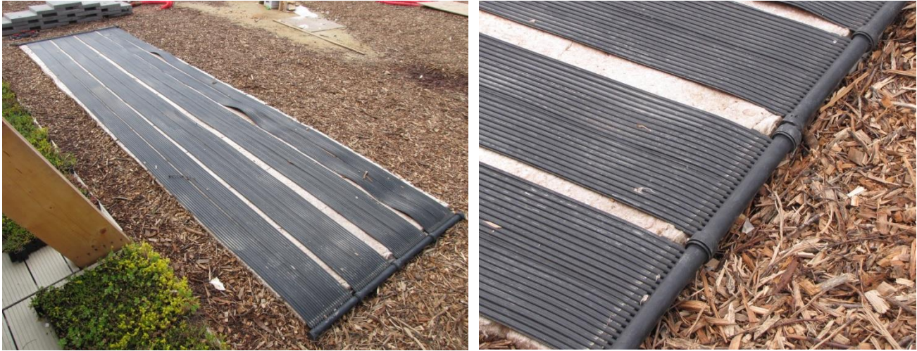
Figure 25 – Views of the unglazed solar collectors installed for EMBRACE
