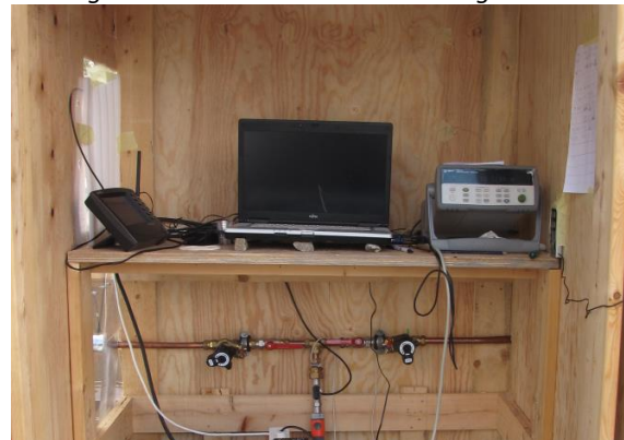
Figure 100 – Datalogging equipment and pipe work
