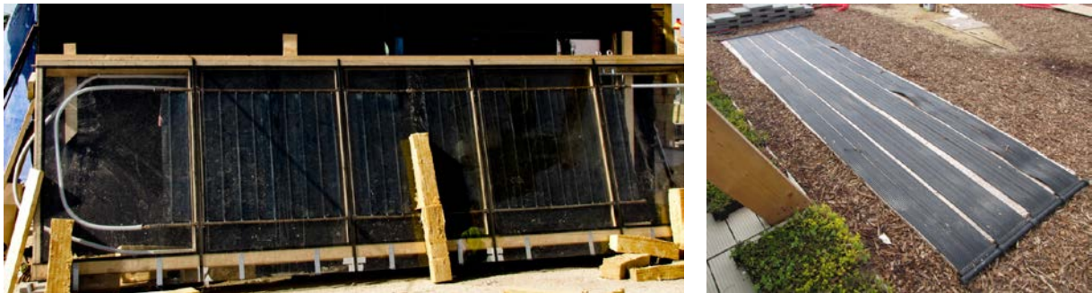
Figure 6. View of the flat-plate thermal collectors before their mounting on the Weather Shield (left), and the unglazed collectors for cooling on the ground (right).
