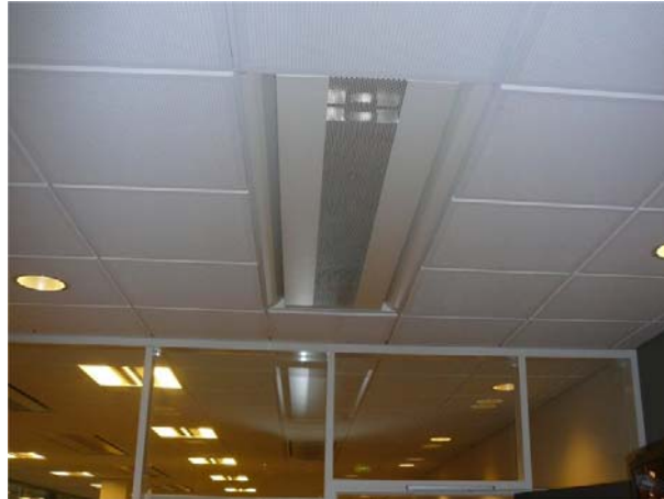
Figure 5: Chilled beams in the office area of the Tuborg Nord [1]
