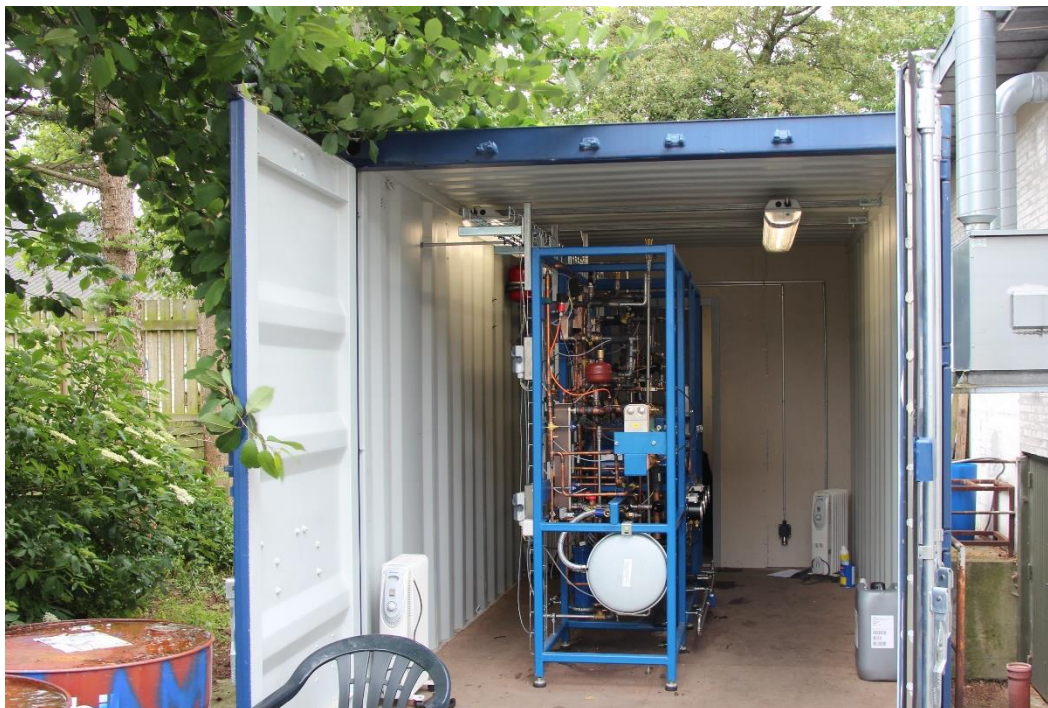
Figur 10b. Varmepumpeopstillingen placeret i container.
