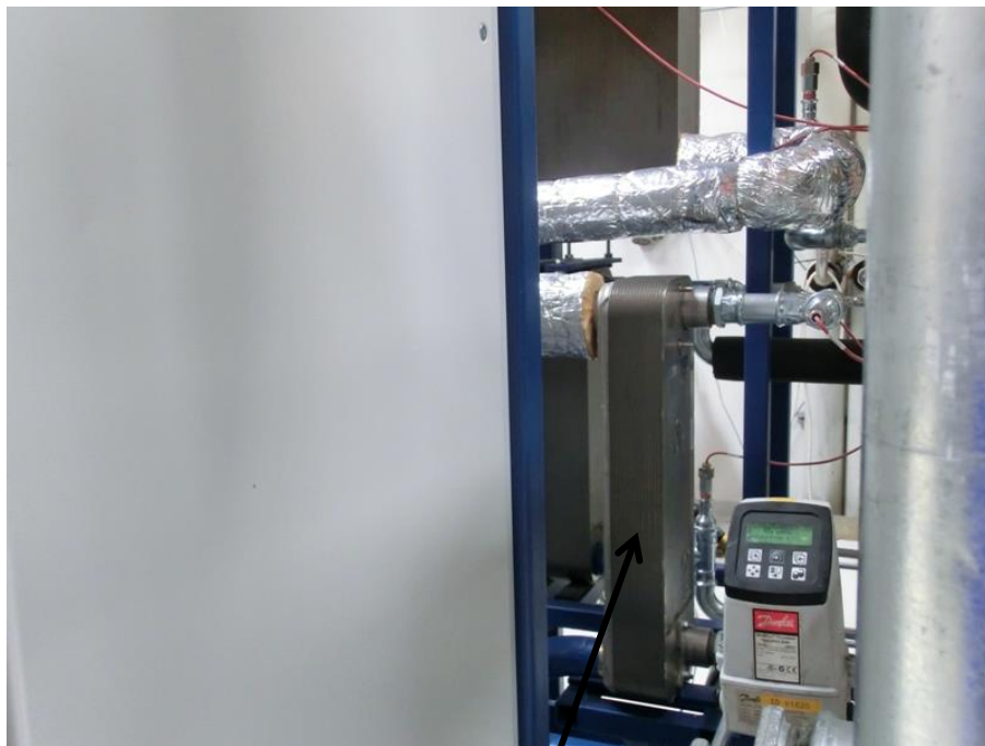
NH 3 sub-cooler Q3
