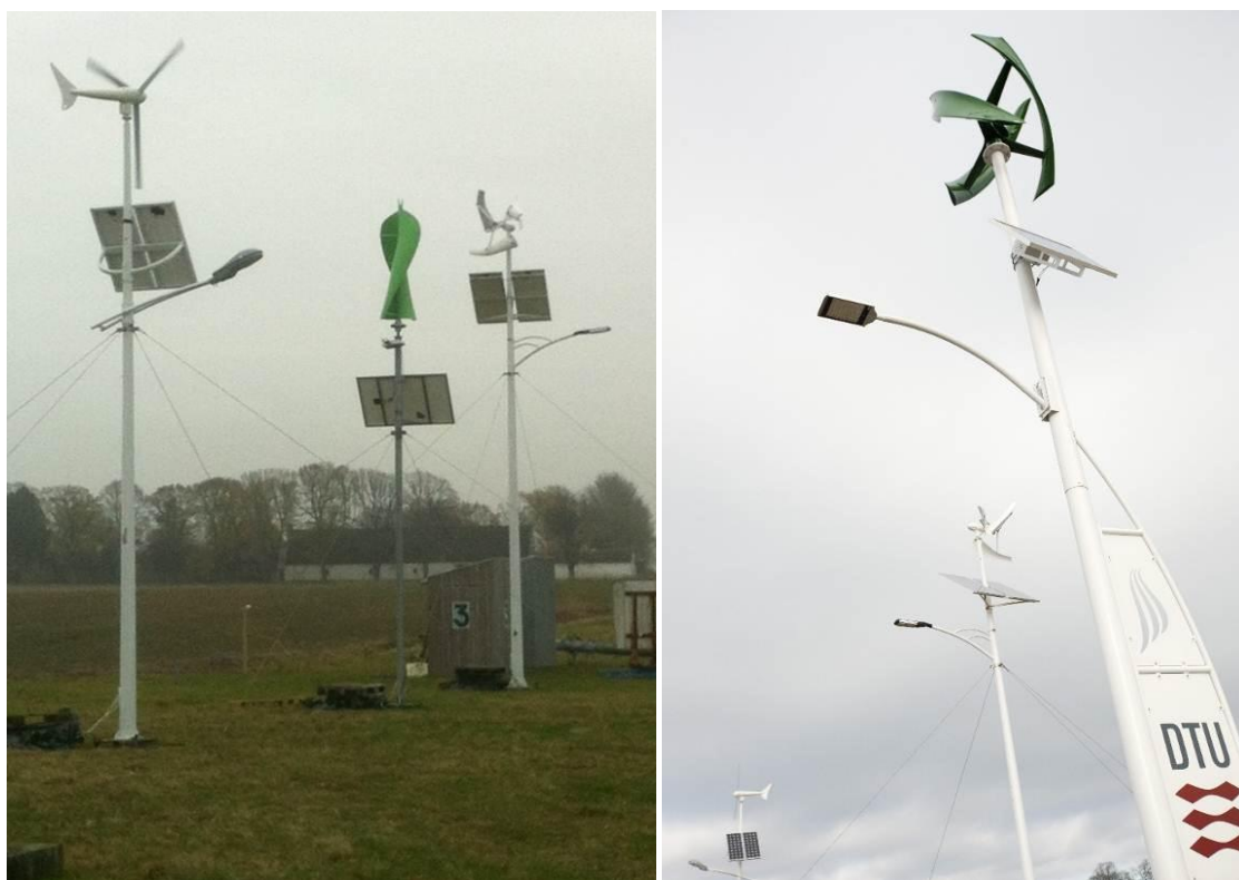
Figure 31 Installed commercial hybrid systems
