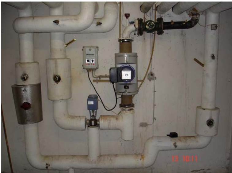
Figur 3.1. Cirkulationspumpen i boilerummet
