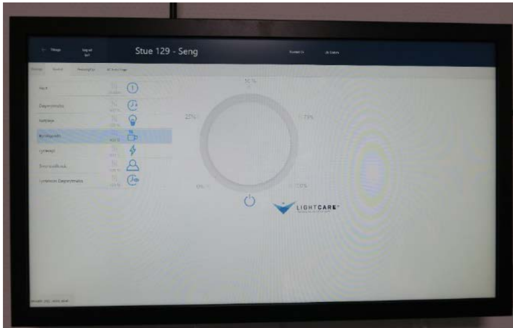
Figure 2-14 - Touch panel for central electric lighting control
