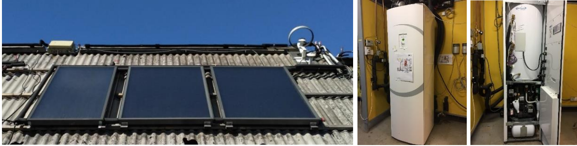
Figure 2. Left: solar collectors. Middle: HYSS system. Right: inside the cabinet of the HYSS system.
