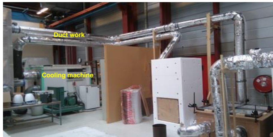
Figure 13 Cooling machine and the duct work
