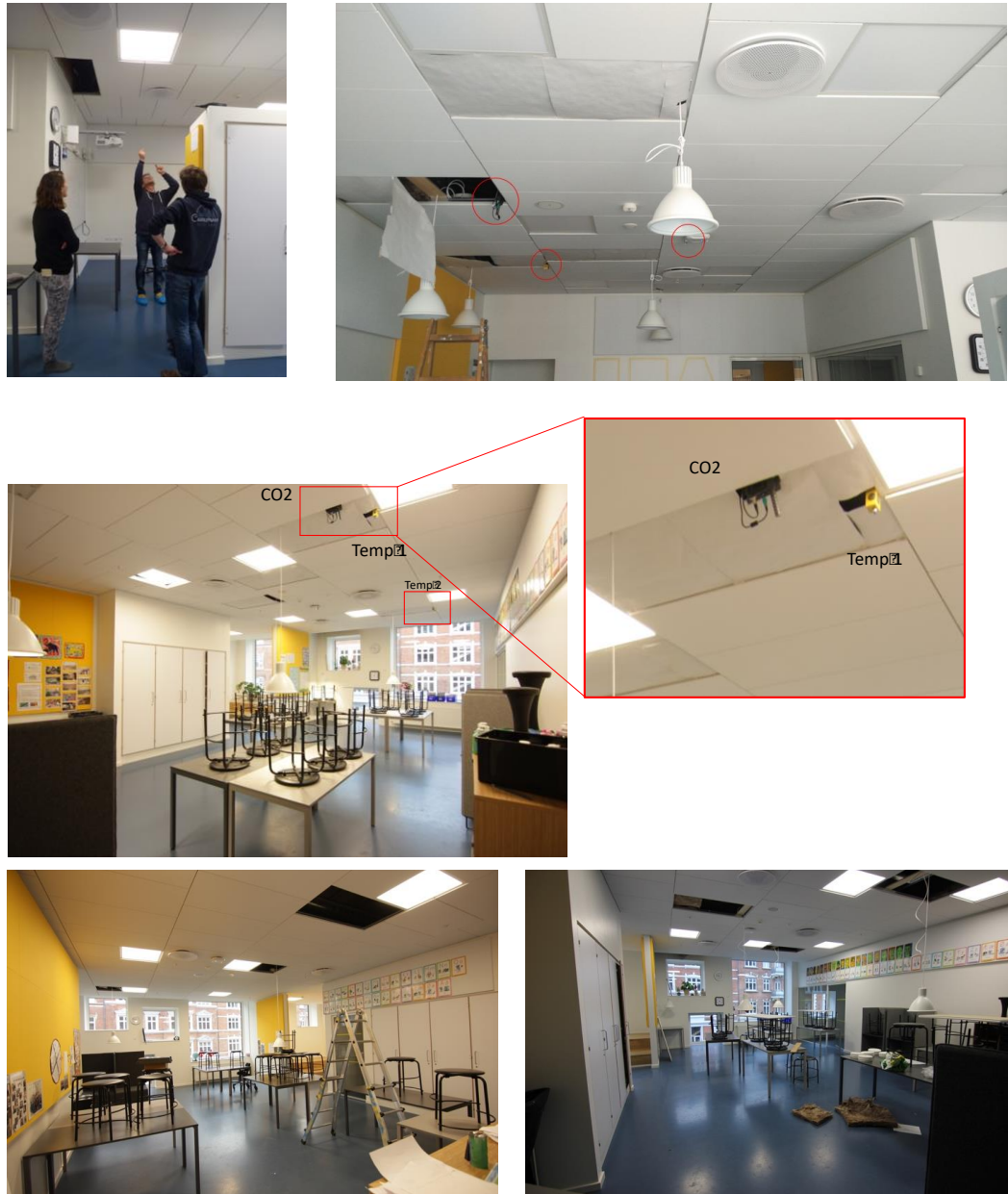
Figure 4.2: Examples of set-up, installation and checking of the indoor climate recording devices
