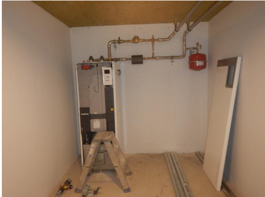
Figur 15. METRO THERM Metrosaver 6 kW MB F varmepumpe under installation i et pulterrum.
