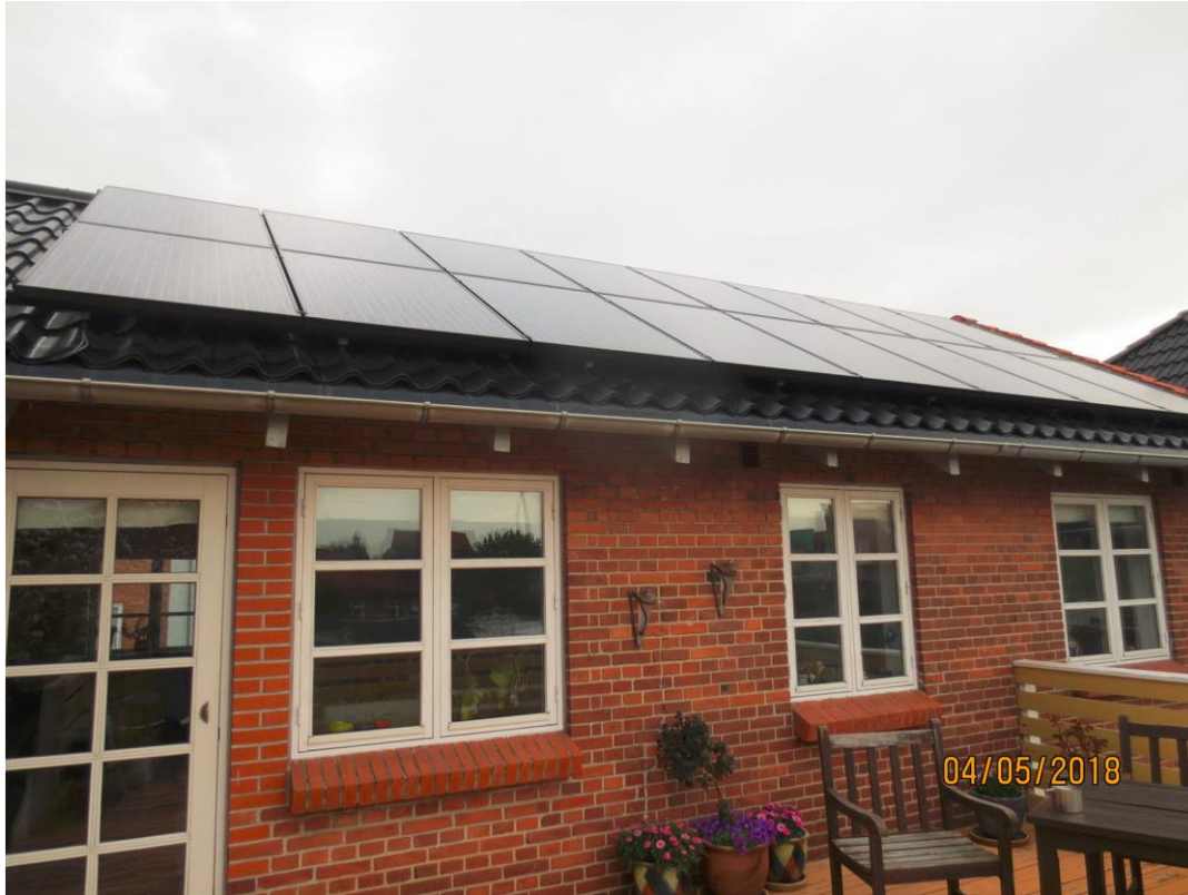
Figure 8. Residential house equipped by solar panels which is located in Esbjerg, Denmark.
